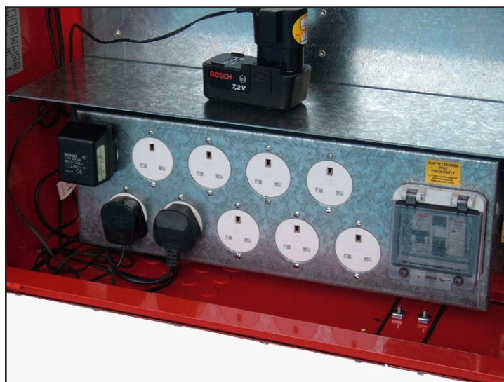
Close up showing MCB, RCD and Sockets
